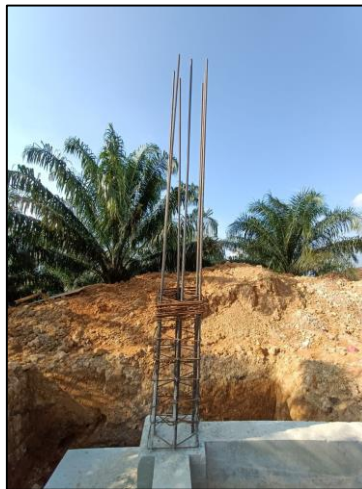
Figure 3.18: Incorrect column rebars
