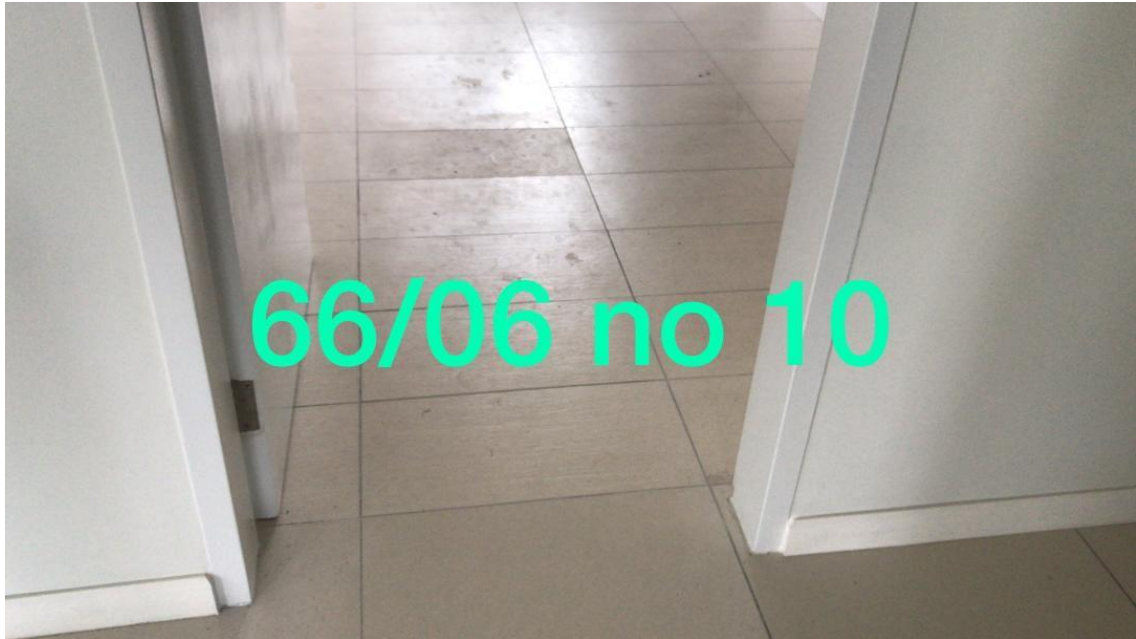
Figure 3.5: Defect Closing Picture.
