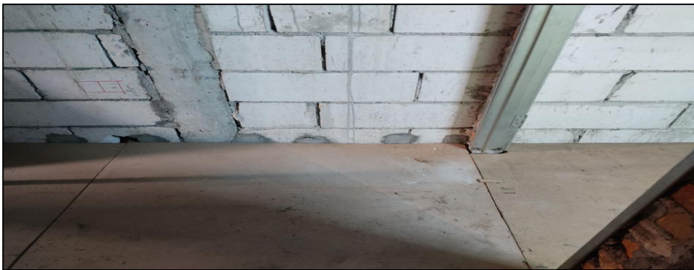
Figure 3.12: First layer of plywood floor that have been installed to floor joist
