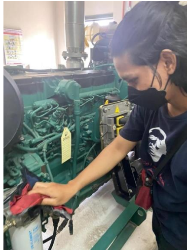
Figure 3.2a service genset monthly
