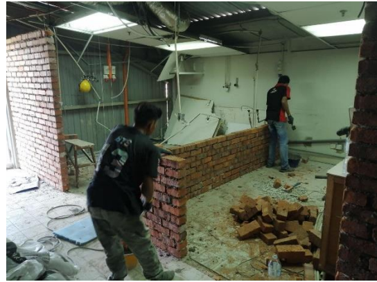
Figure 4: The construction of clay brick walls at Autoclave Lab and Centrifuge Lab
