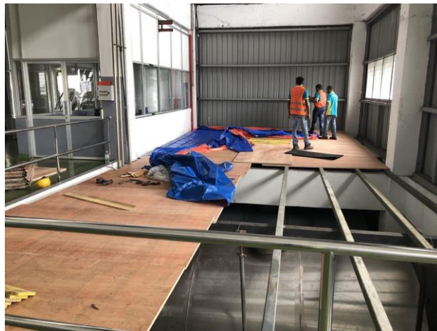
Figure 3.13 shown the labours laying the plywood on top of the hollow steel structure
