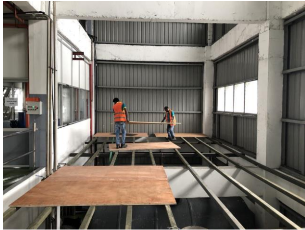
Figure 3.12 shown the labours laying the plywood on top of the hollow steel structure
