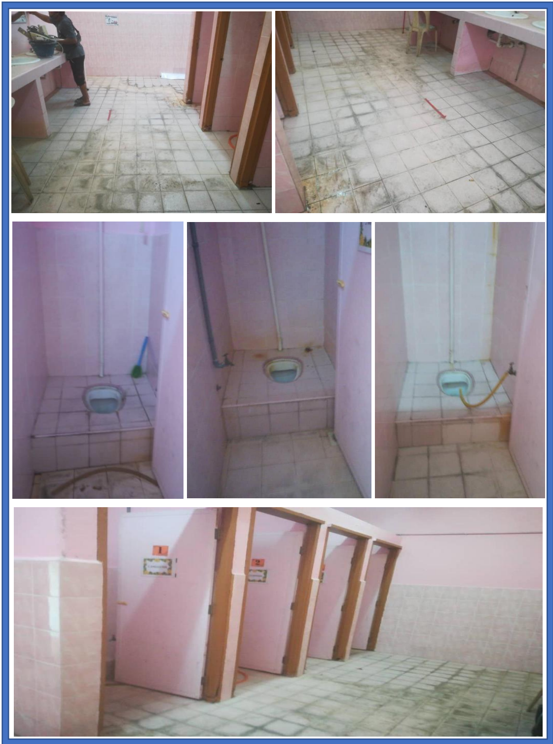
Figures 3.3.1: The condition of the toilet's tiles, cubicles, and doors.
