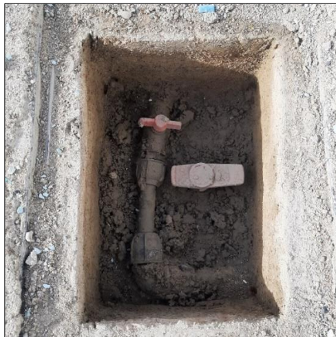
Figure 3.10: freshwater pipelines to the pool
