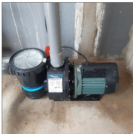
Figure 3.29: pump used for above ground level swimming pool
