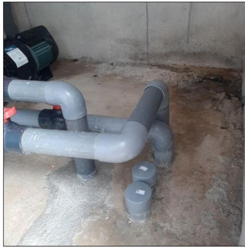
Figure 3.9: Connection of PVC pipe with PVC ball valve in pump room
