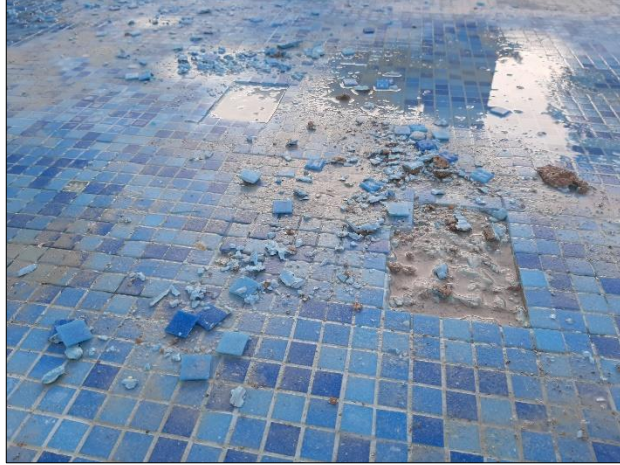
Figure 3.35: Certain part of installed mosaic tile start falling off
