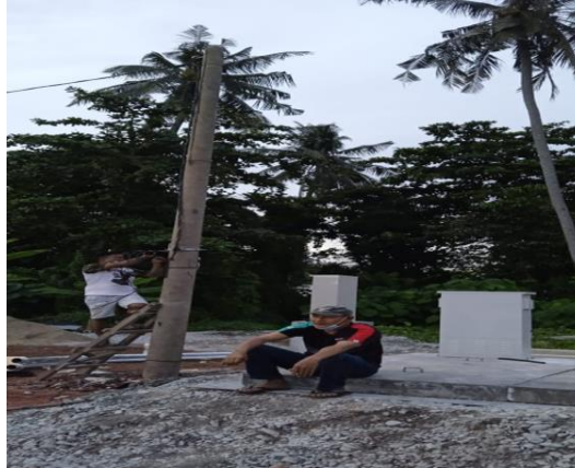
Photo 3.3.11 TNB worker installing grounding pole and bypass the electricity from street light
