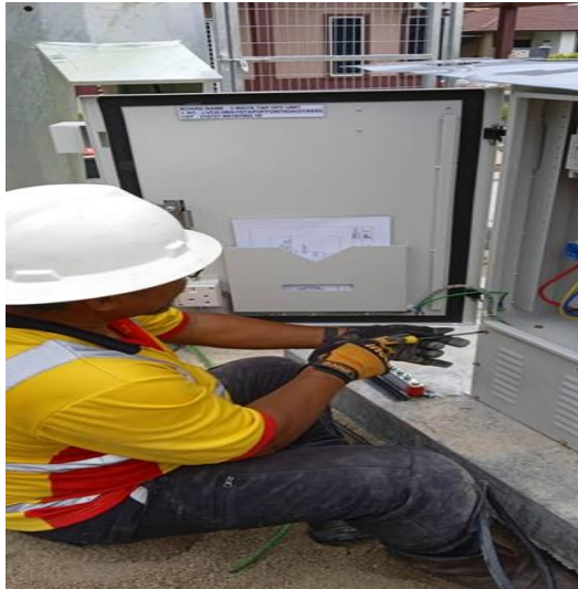
Photo 3.3.23 Wiring at bottom for electric box
