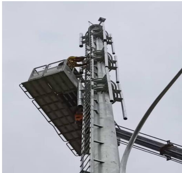
Photo 3.3.22 Wiring at top TLP for boom
