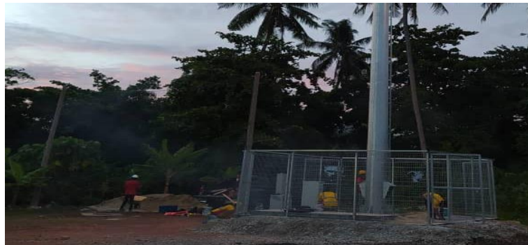
Photo 3.3.27 Cleaning up the site and fill the surrounding with sands and pebbles
