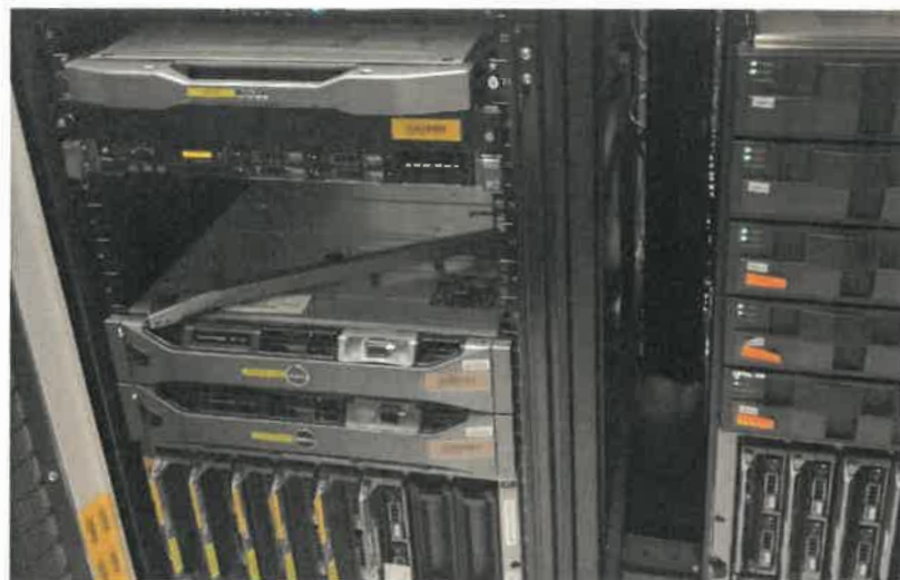
Figure 9: Data Centre Unit Site Visit
