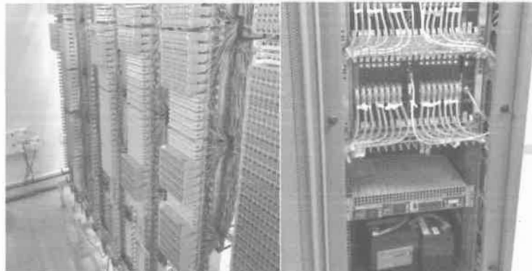
Figure 15: Communication Unit Site Visit
