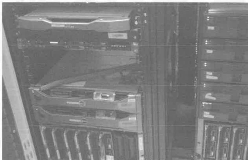
Figure 9: Data Centre Unit Site Visit
