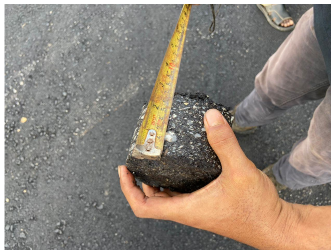
Figure 3.3.2 The worker is measure the part of compacted premix that have been taken from coring test
