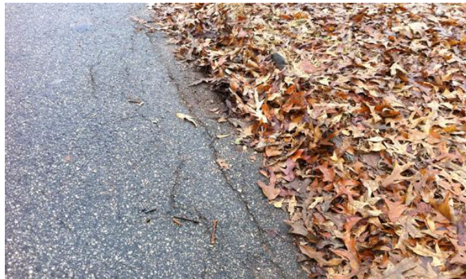
Figure 3.4.5 Road with Edge Cracks
