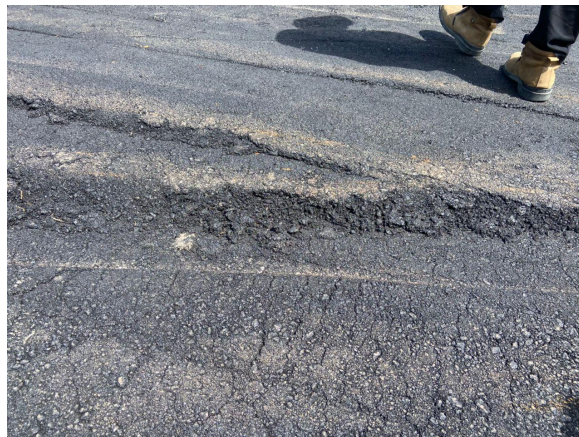
Figure 3.4.8 Road with Rutting Cracks
