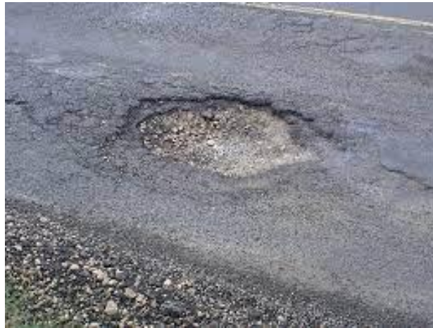
Figure 3.4.7 Road with Pot Holes Cracks
