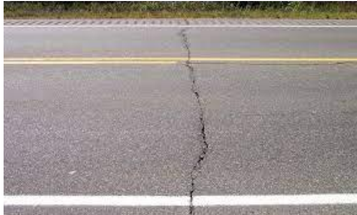
Figure 3.4.4 Road with Transverse Crack
