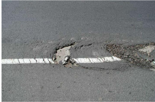
Figure 3.4.6 Road with Slippage Cracks
