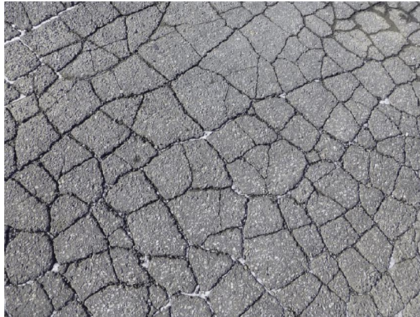
Figure 3.4.1 Road with Alligator cracking
