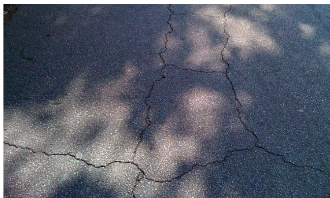
Figure 3.4.2 Road with Block Cracking
