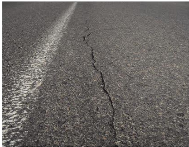
Figure 3.4.3 Road with Linear Cracking
