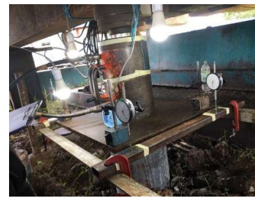
Setup for dial gauge and mechanical hydraulic mechanical pump for Maintain Load Test
