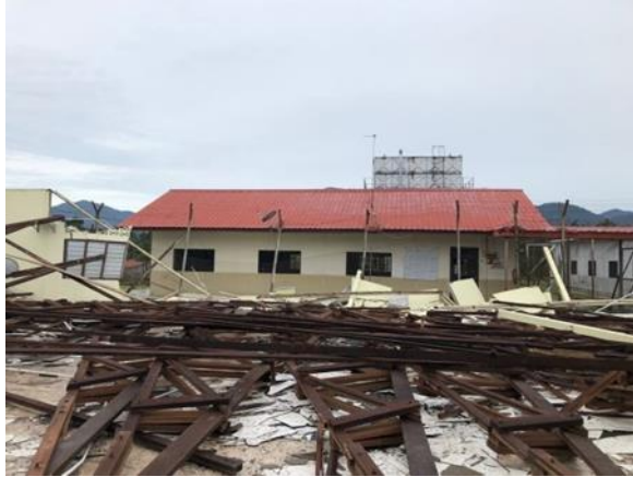
Figure 24 The condition of the joist and trusses that have fallen
