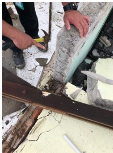
Figure 25: Beam foundation condition
