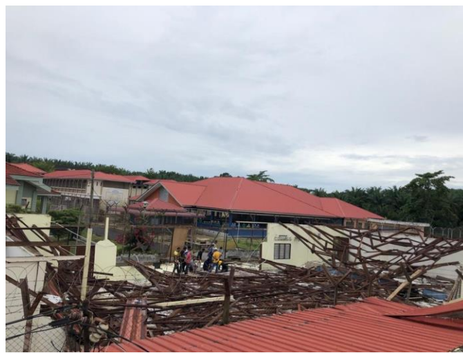
Figure 7 The overall view from the top of the collapsed hall building
