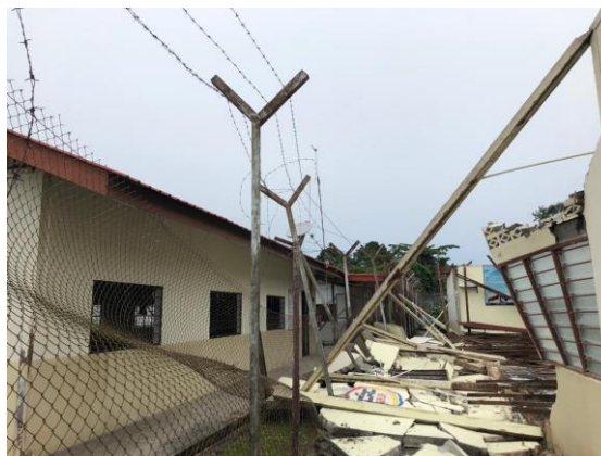
Figure 9 The condition of the fallen wall
