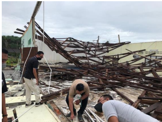
Figure 8 Inspection activities of the hall that have fallen and collapsed
