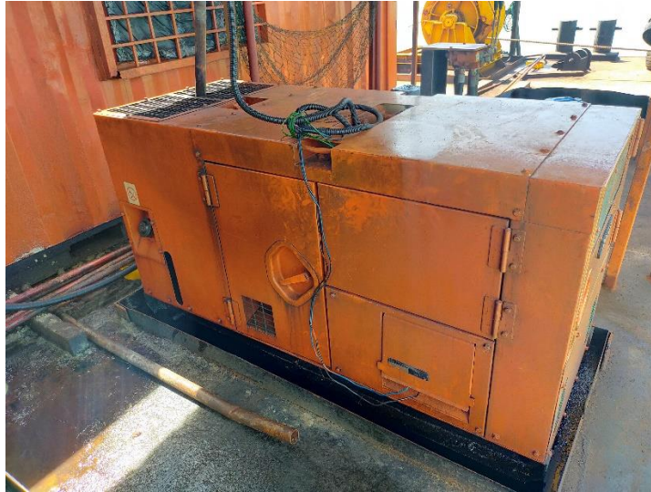
Figure 3.3.5 Genset as power supply Source: Observation (camera phone)
