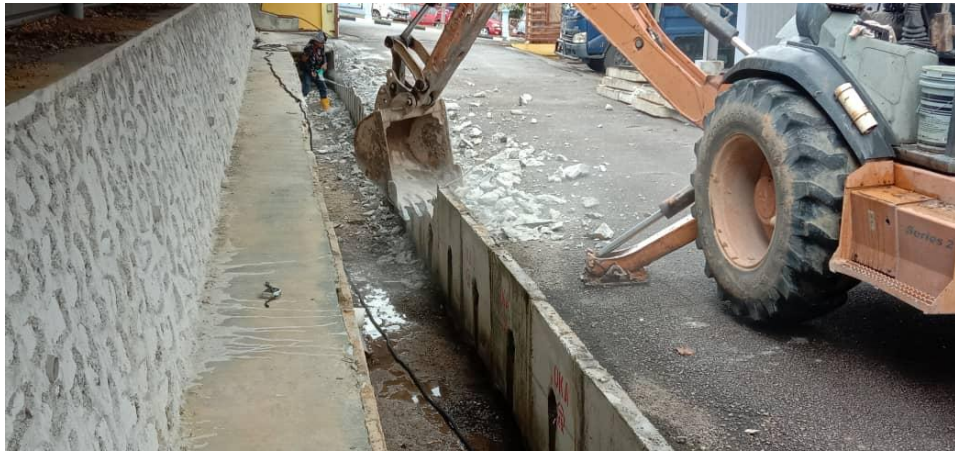
Figure 1.18: Breaking part of the culvert concrete drainage
