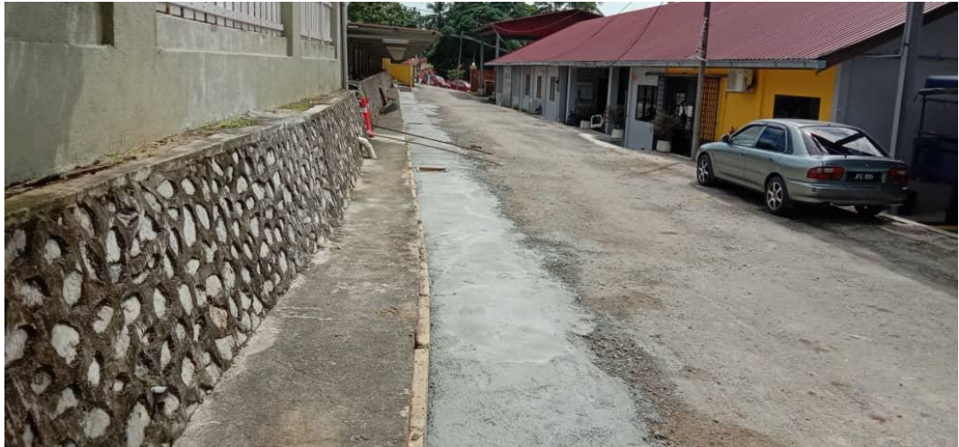
Figure 1.23: concrete mix above culvert drain box
