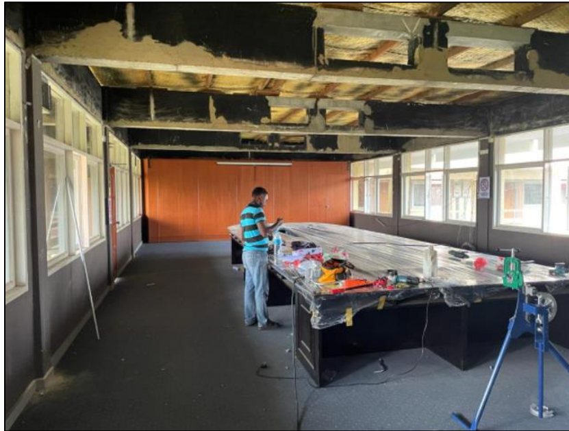
Figure 3.23: The fault of the worker doing the work in the incorrect place
