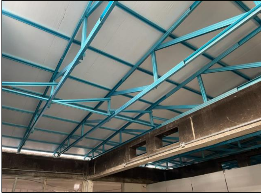
Figure 3.19: View of the project after being installed with the new roof trusses
