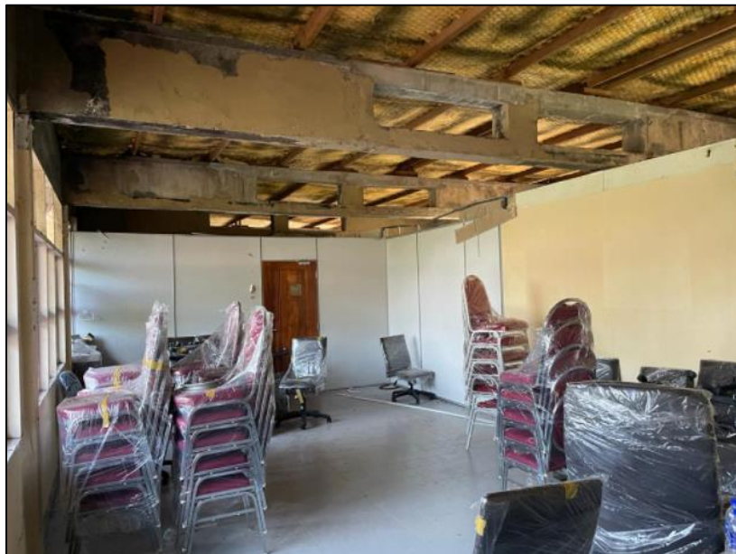
Figure 3.22: All furniture is being wrapped to avoid the rainwater and sunlight from hitting the surface of the furniture
