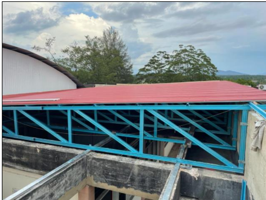
Figure 3.20: View of the project after installation of the new metal deck roofing sheets
