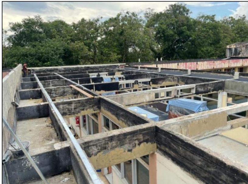
Figure 3.16: View from the top after dismantling the roof trusses and roofing sheets
