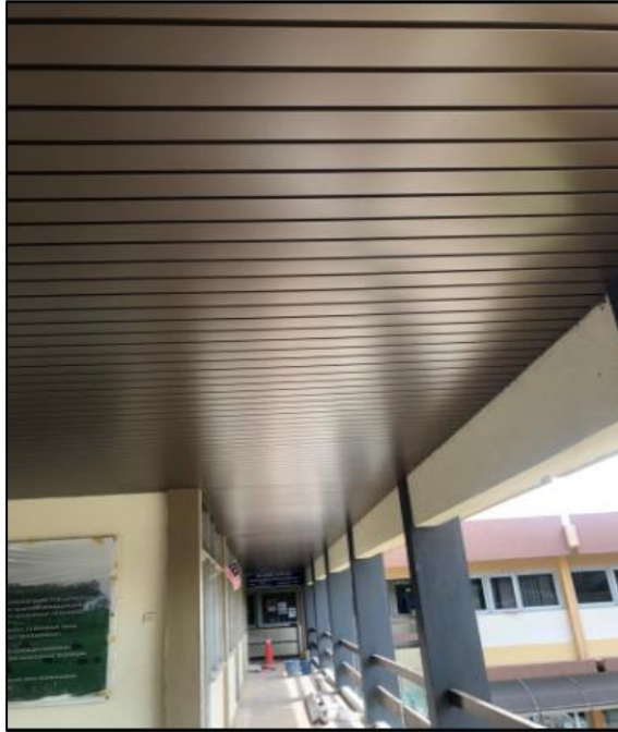
Figure 3.21: View of the project after the installation of the aluminum strip ceiling
