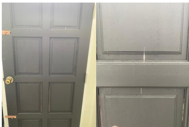
Figure 3.27 Holes at door.
