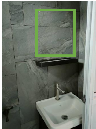
Figure 3.31 Toilet window broken.
