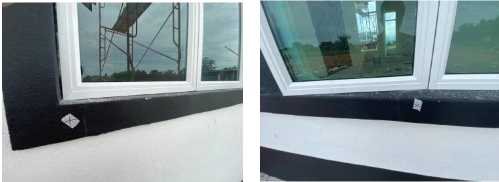
Figure 3.28 Window cannot open because of coping
