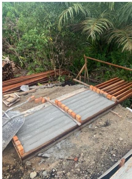
Figure 3.2.7(b) The pre cast lintels that been used at the bottom and top of opening part
