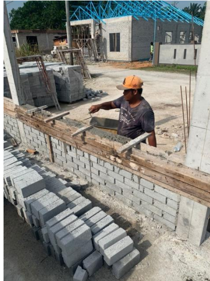
Figure 3.3.4 lintel beam are being made in-situ with cement, sand and gravel mix
