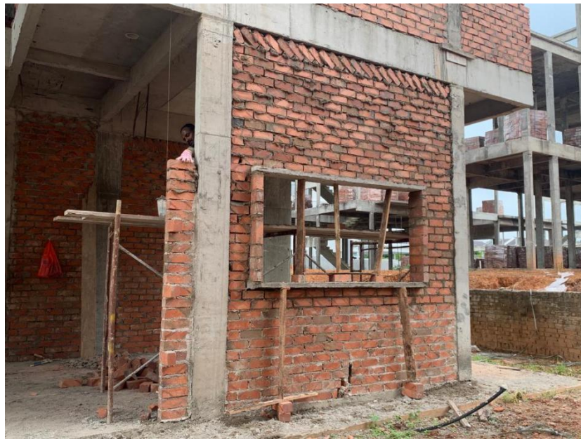
Figure 3.2.10: The lintels that used as a load support at the top of opening parts.
