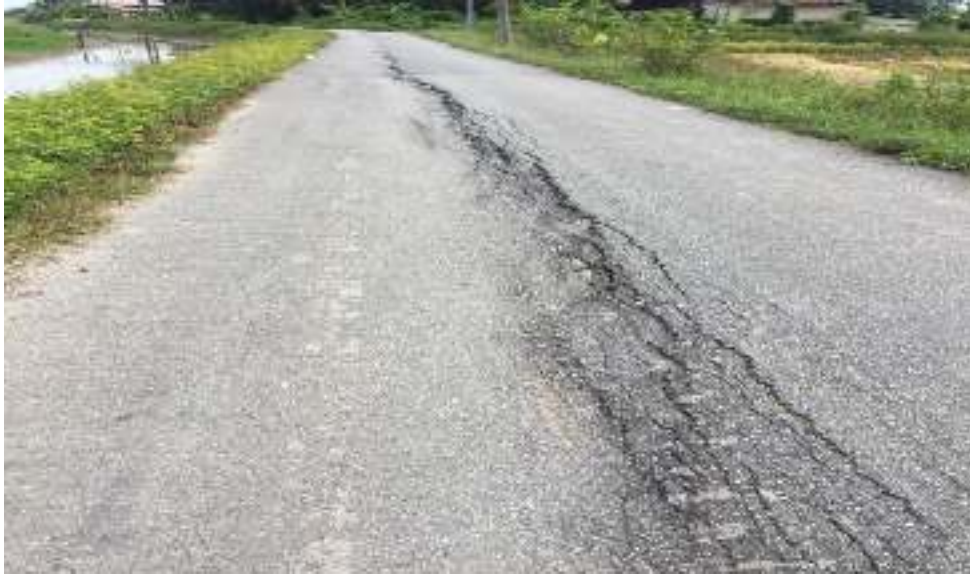
Figure 3.2: Depression of road
