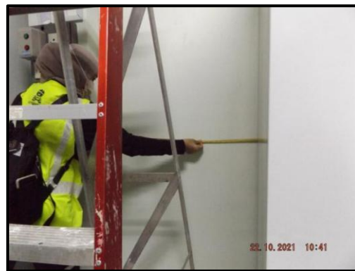
Figure 3.21 : Measuring The Defect Length
