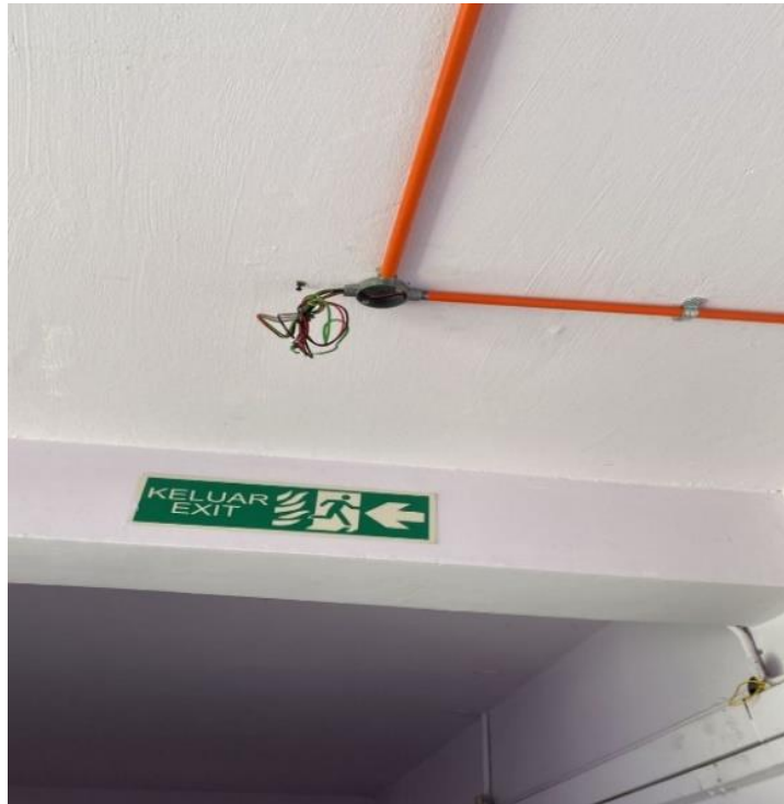
Figure 3.3.4 : excess dangling wire.
