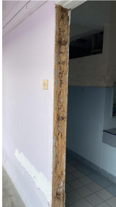
Figure 3.3.6: No door and frame has been eaten by termites at toilet door Cemara B
