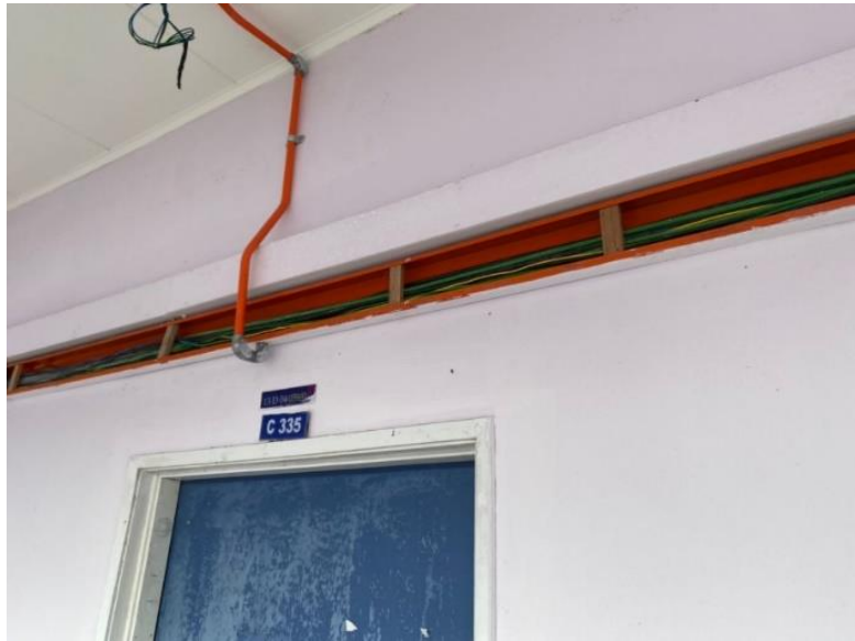
Figure 3.3.3 : The steel panel Cover for the wire missing
