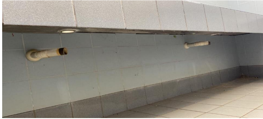
Figure 3.3.2: The bottle trap is not installed or has been remove.
