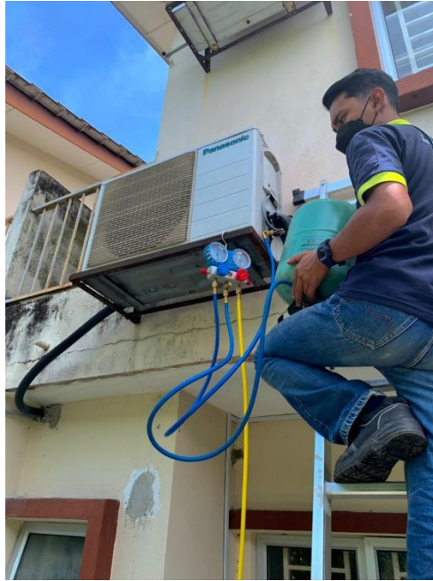
Figure 3.3: Fixing on the leak of AC refrigerant
