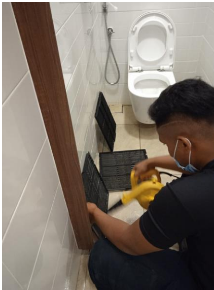
Photo 3.4.5: Dry the air filters
