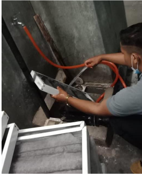
Photo 3.2.4: Clean the AHU air filters
