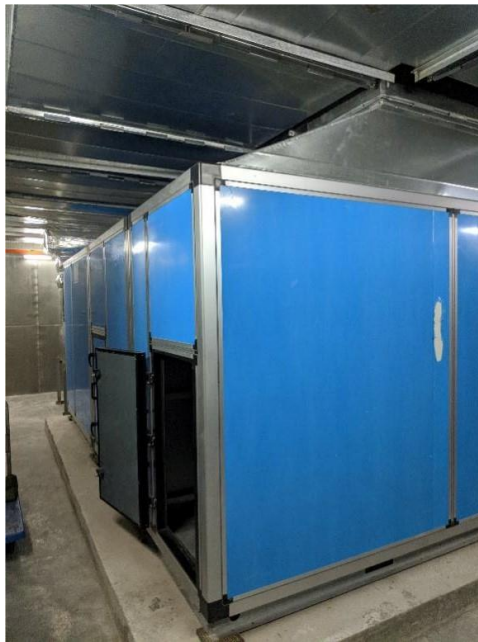
Photo 3.2.7: Close back the AHU door
