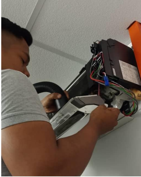
Photo 3.3.4: Suck stagnant water
