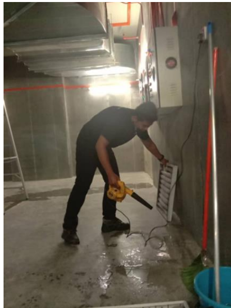
Photo 3.2.5: Dry the air filters
