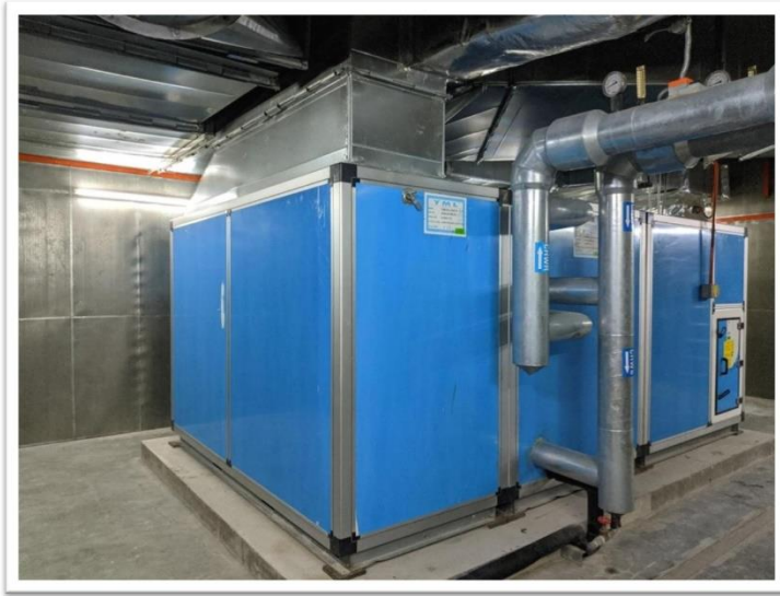
Photo 3.2.2 Air Handling Unit (AHU)
