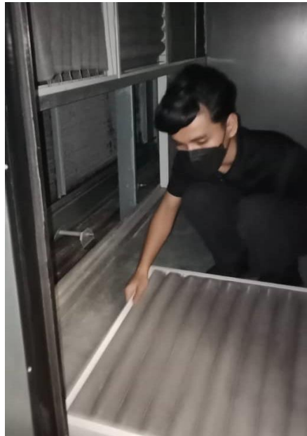
Photo 3.2.3: Take out the air filters
