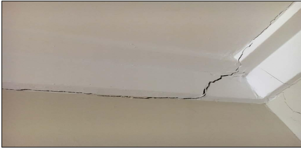
Figure 3.20: The delamination crack.
