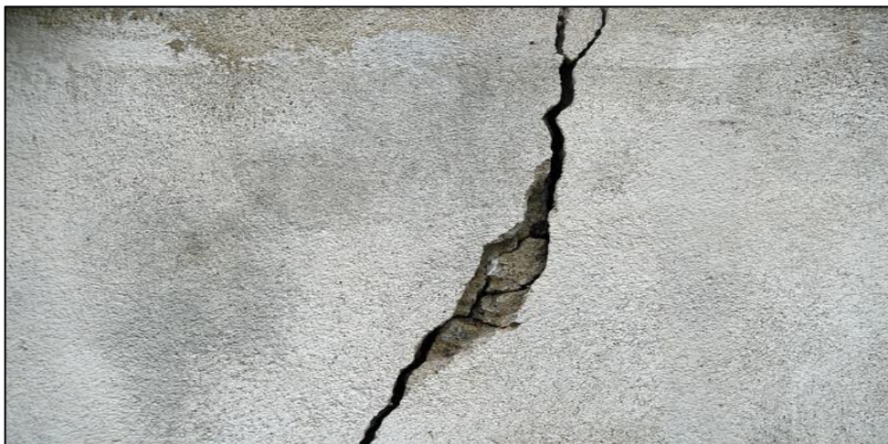
Figure 3.19: The settlement crack. (Source: https://cutt.ly/5TevOtc )
