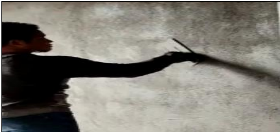
Figure 3.14: The finishing trowel was used to make sure the coat of the concrete is smooth.
