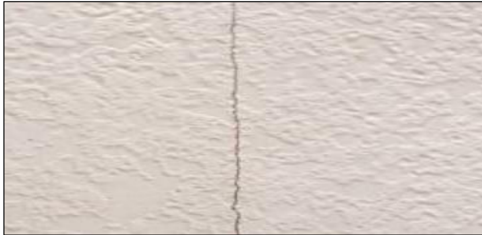
Figure 3.18: The hairline crack. (Source: https://cutt.ly/WTcvbfu )
