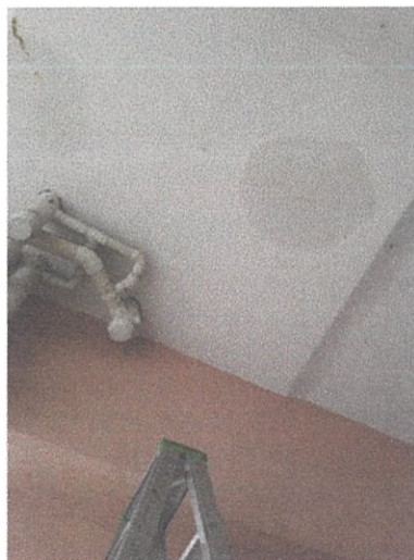
Photo 3.13: leaking on floor slab
