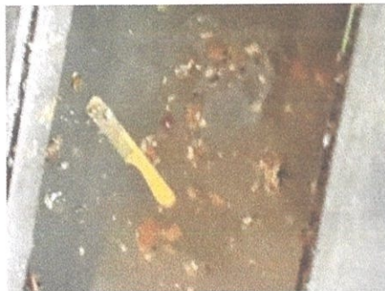
Photo 3.1: garbage and debris blocks the sewage
