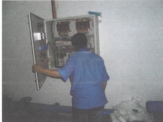
Photo 3.21: checking control panel
