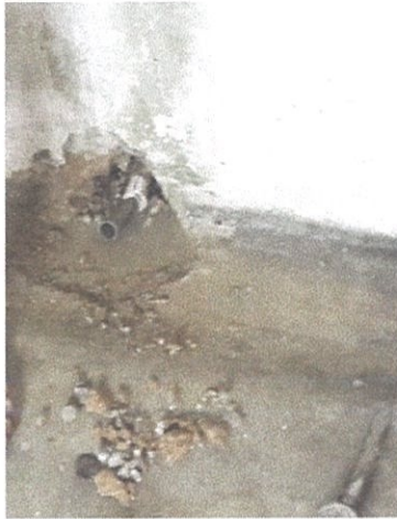
Photo 3.16: drain hole for corridor
