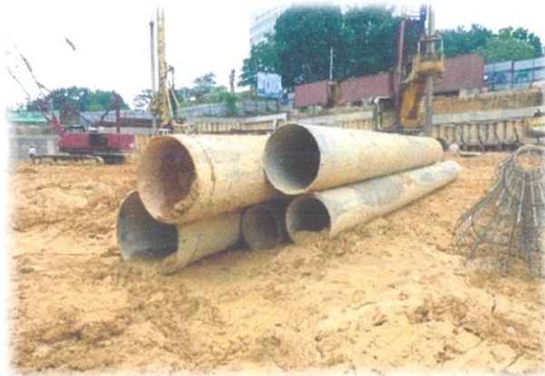
Photo 3.15: Temporary steel casing will be installed before the drilling work is done
