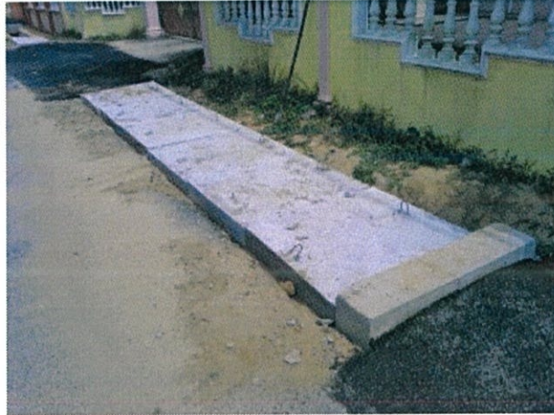
Figure 3.3 Drain closure plays an important role for the safety of road users
