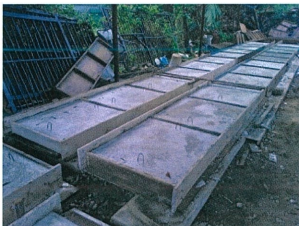
Figure 3.24 Concrete is hard and sturdy after hardening process
