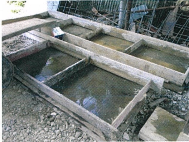
Figure 3.17 Picture of moistured formworks
