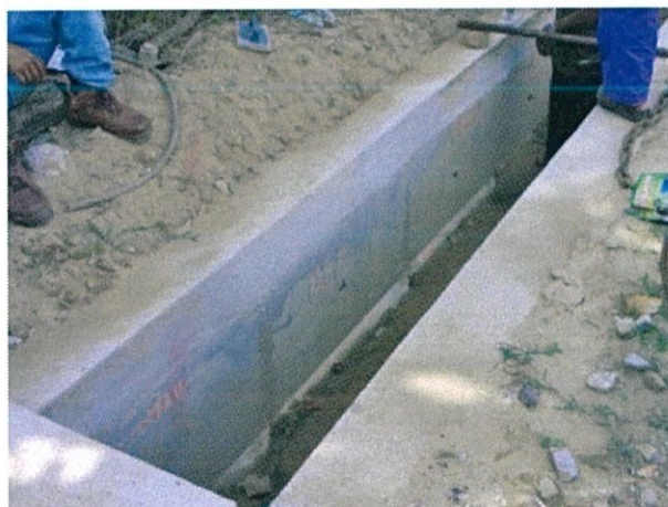
Figure 3.2 The exposed drain could lead to dangers to people
