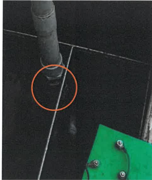
Figure 19: The broken valve
