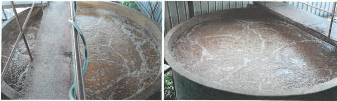
Figure 2: Aeration tank 1 (left), Aeration tank 2 (right)
