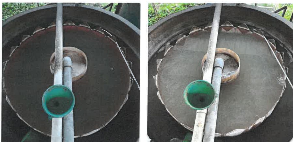
Figure 11: Primary clarifier tank on 14 th July 2022 (left) and 24 th May 2022 (right)
