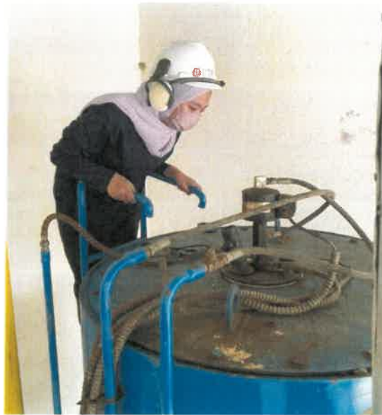
Appendix 17 : Trainee run the boiler under En. Azlan supervision.
