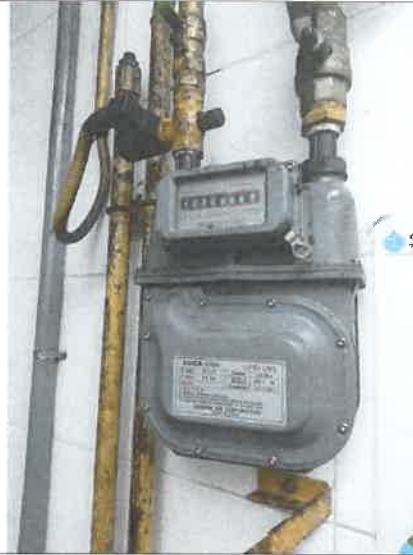
Meter Reading At Malls
