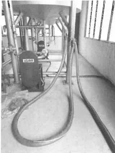
Figure 6: PVC pipe that were used to transfer the base oil from storage tank to IBC, from IBC to mixing tank
