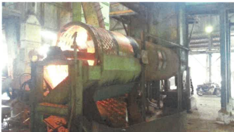
Figure 25: Polishing drum in mill
