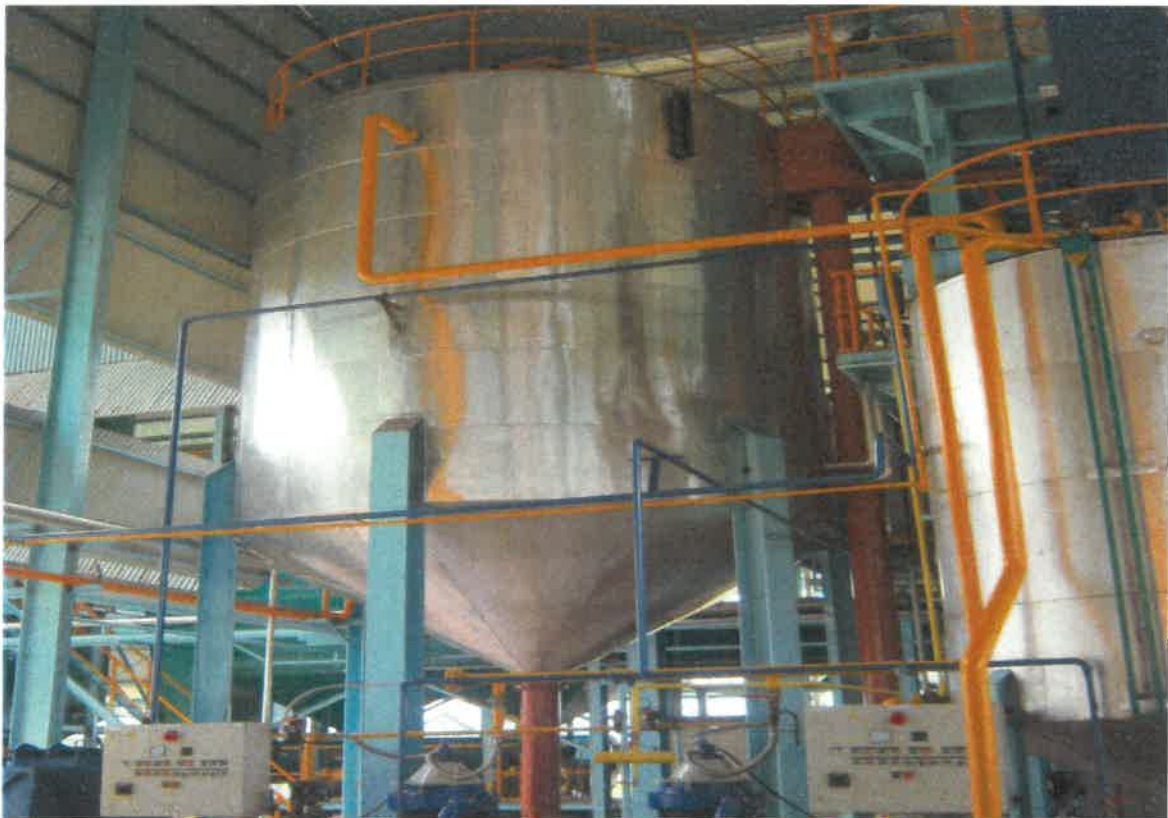
Figure 18: Settling Tank in Mill
