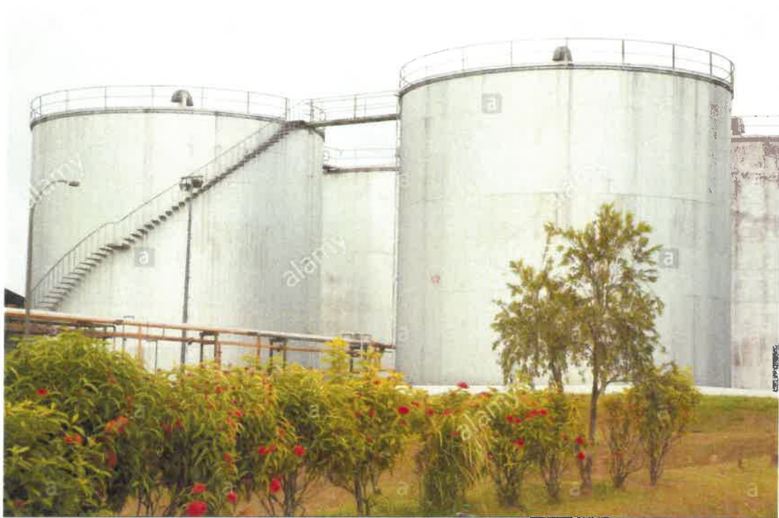
Figure 22: Storage Oil Tank
