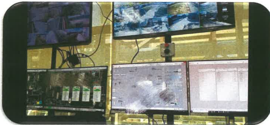
Figure 18. Checking data through Programmable Logic Controller
