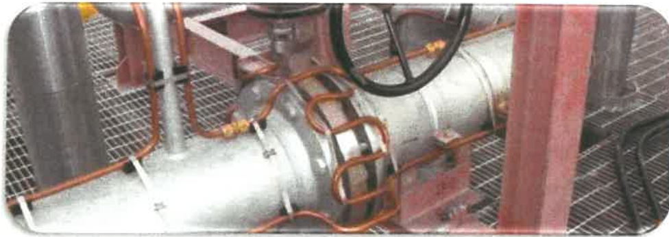
Figure 24. One of piping with steam tracing
