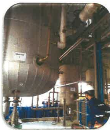
Figure 27. One of the equipment that undergoes flash vaporization
