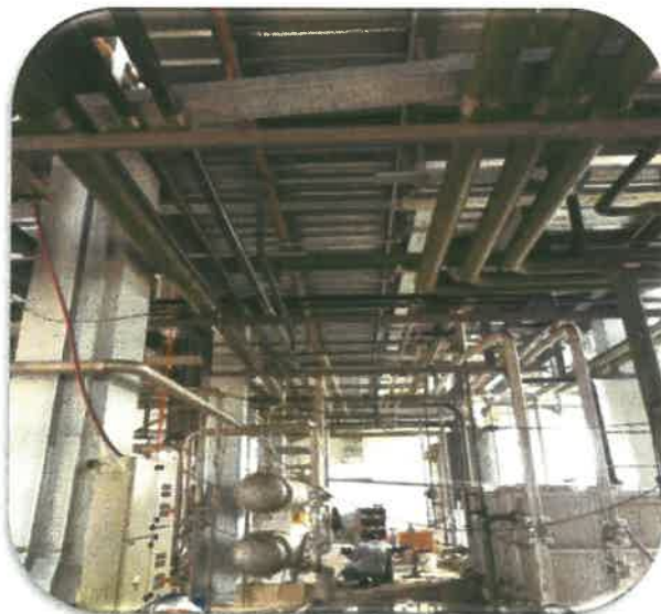
Figure 20. View of piping and instrumentation in the plant
