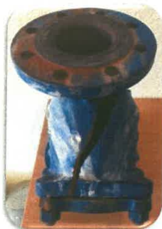
Figure 26. Steam hammering effect on pipe
