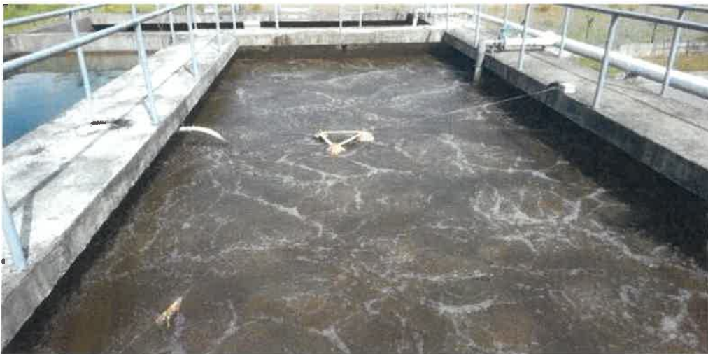
Figure 9: Aeration Tank of the Wastewater Treatment System at Halal Abattoir Complex
