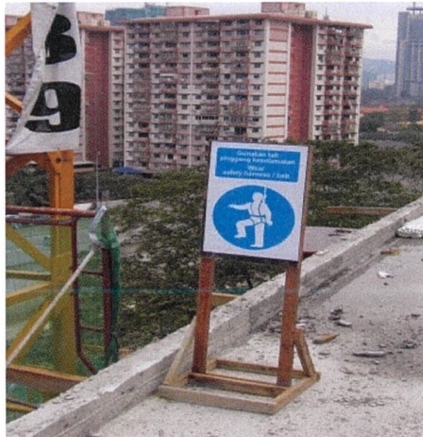
Photo 3.3.8: Safety harness signage.
