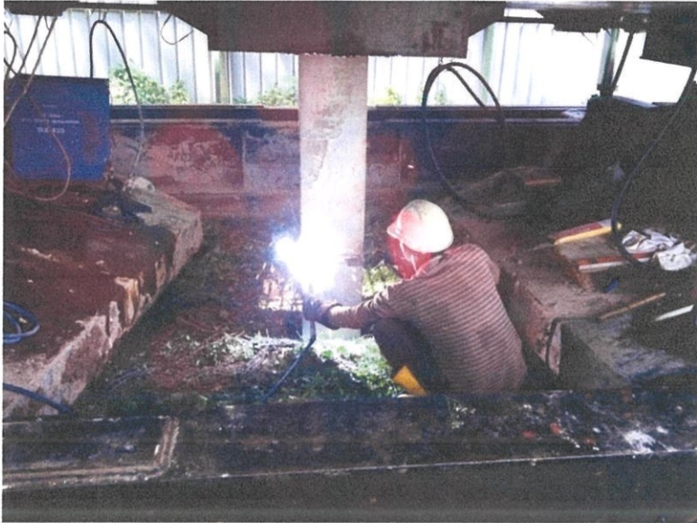
Figure 3.3.15 : the pile will be welding if the use of piling more than 1 in single point.
