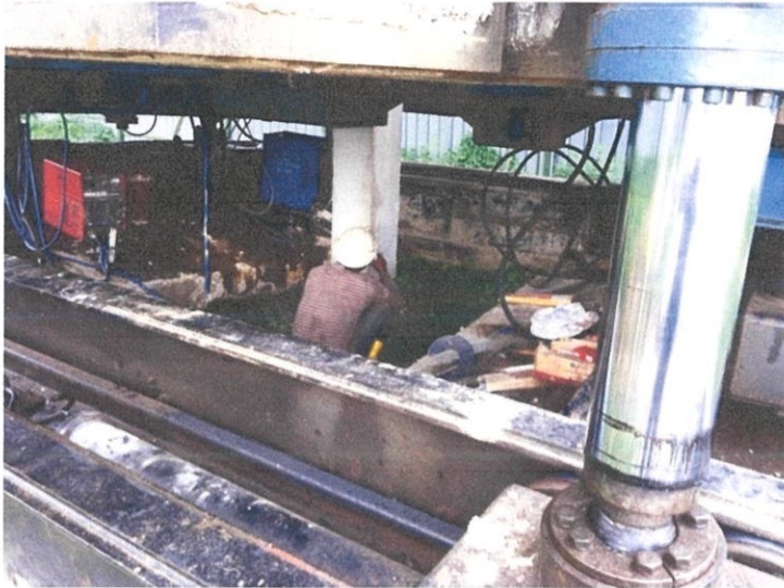
Figure 3.3.13 : the worker was measuring the depth of pile that has been forcing down until it reached the maximum penetration.
