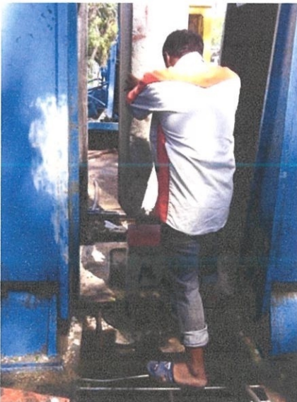
Figure 3.3.12 : pile is forcing down to the ground by using the jack-in machine.
