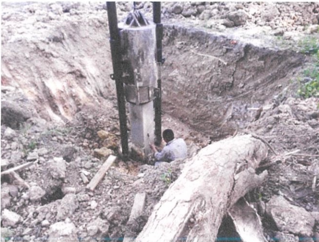
Figure 3.3.16 : the worker taking the result and measure the strength of pile, if the pile cracked, then it will be remove and change with another pile
