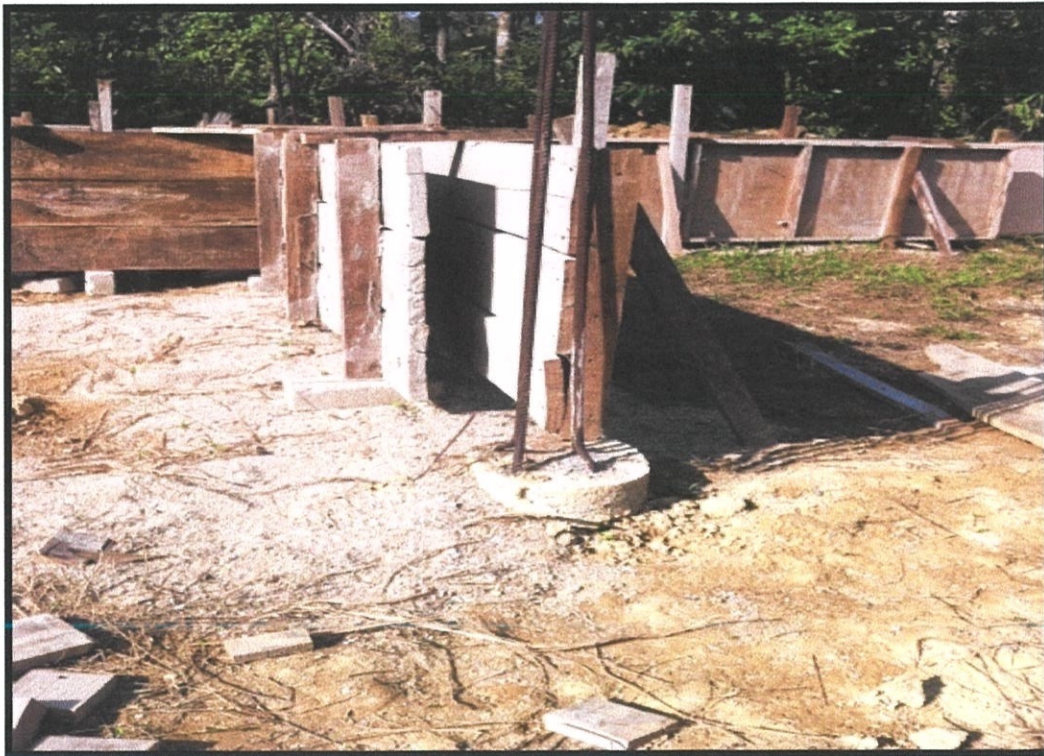
Figure 3.4: Installation formwork for ground beam is doing and used support wood to avoid formwork from falling down.
