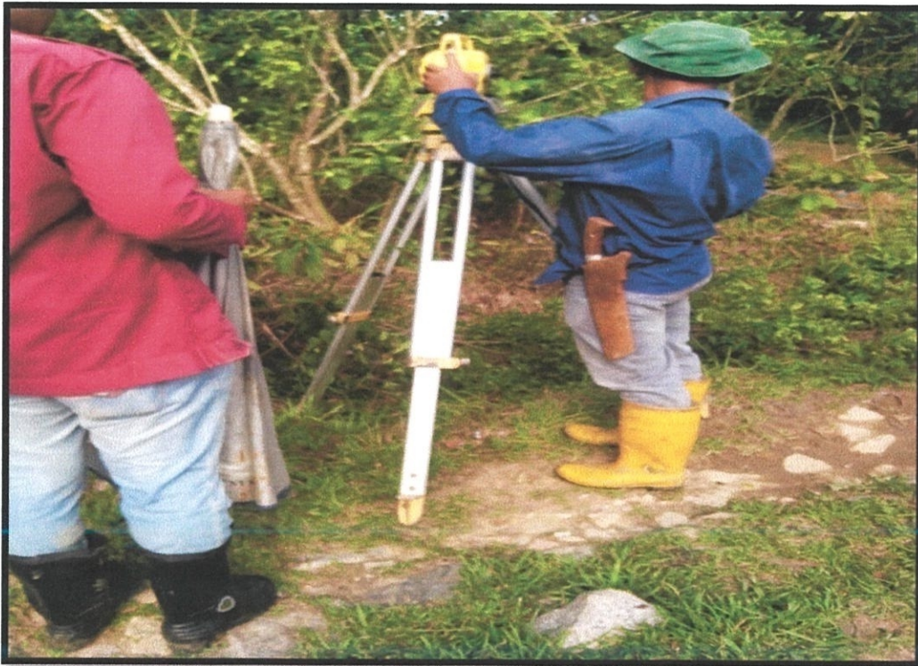
Figure 3.1: Setting out work to get mark and line to determine position at ground floor.
