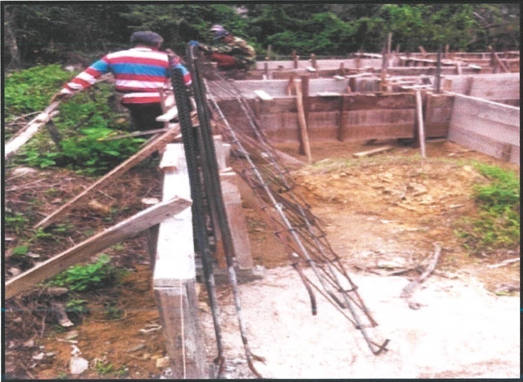
Figure 3.5: Installation reinforcement bar for ground beam after formwork done to install, type for reinforcement bar used is Y16.
