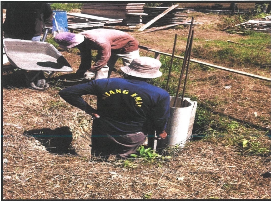
Figure 3.3: The installation formwork for footing and infill concrete into formwork in doing by using wheelbarrow.
