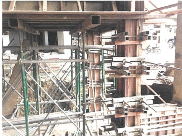
Picture 3.19: Wrong size of stiffener need to be open
