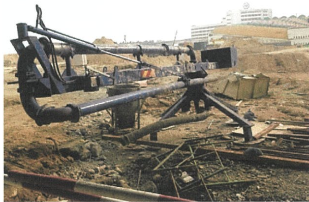
Picture 3.23 : Spider machine broken
