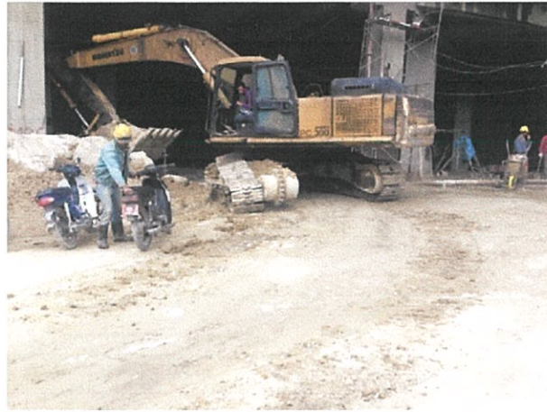
Picture 3.21 : Excavator accidently hit staircase
