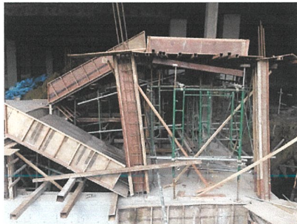
Picture 3.22 : Staircase were hitted
