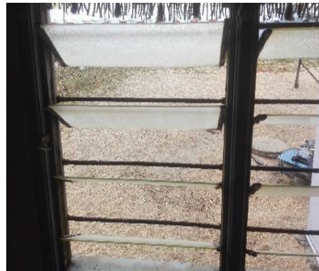
Corrosion of Louver windows
