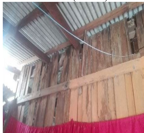
Decay on the timber wall and sticky surface (sea salt).
