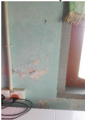
Peeling of the paint due to dampness and sticky surface (sea salt)
