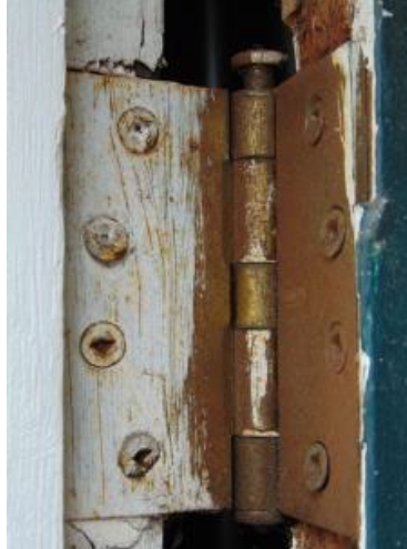
Corrosion of Door Hinge
