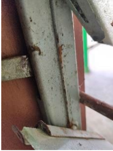
Corrosion of Louver windows
