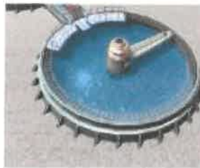
Figure 6. Circular basin in water treatment industry
