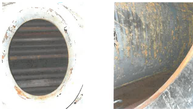
Figure 6: (a) Fire side of boiler
