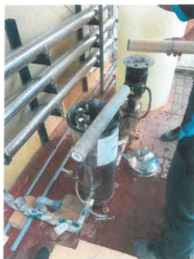
Figure 19. Troubleshooting process of reverse osmosis system.
