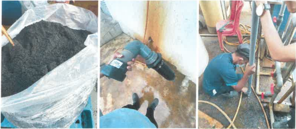
Figure 17. Process of changing activated carbon for Activated Carbon Filter.
