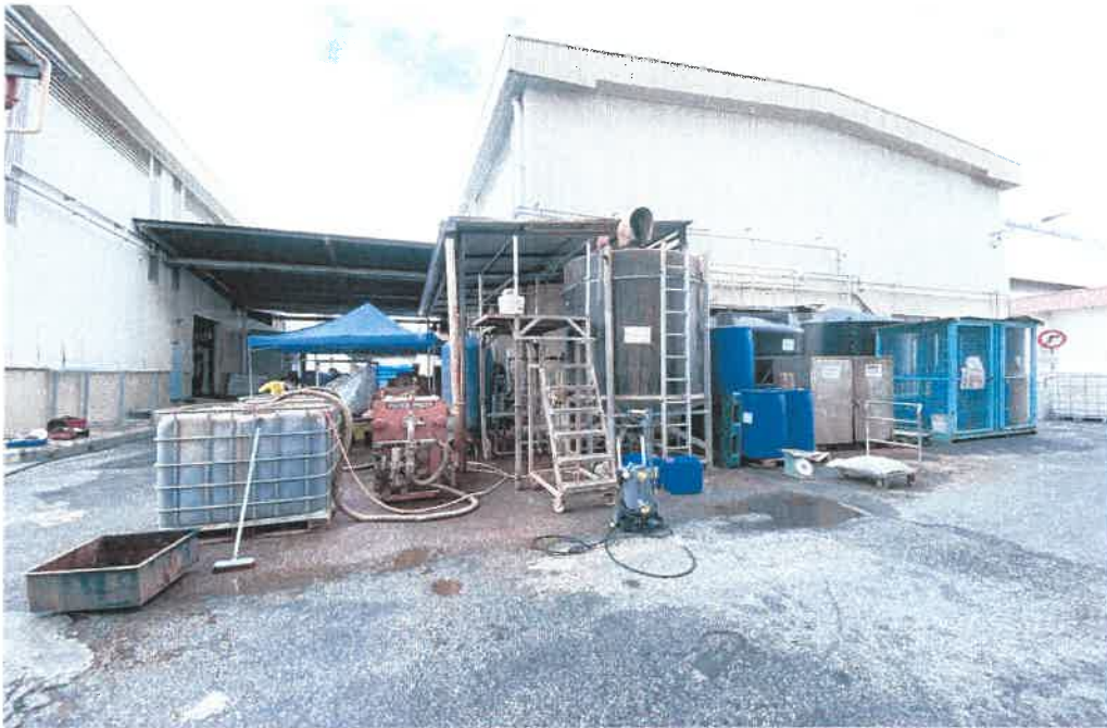
Figure 19: Matrix's Temporary Wastewater Treatment Plant
