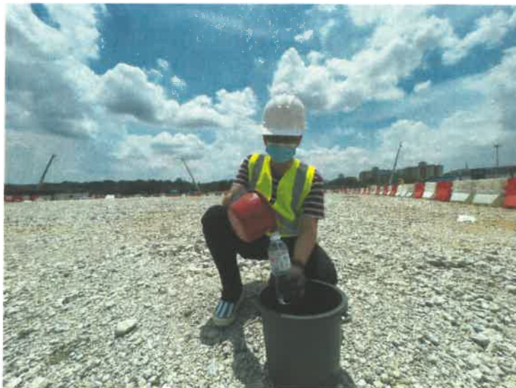
FIGURE 15: RAIN WATER SAMPLE COLLECTION IN MRT BANDAR MALAYSIA
