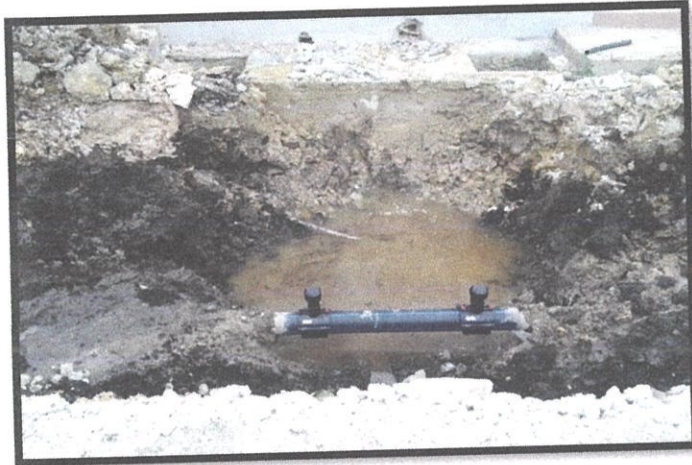
Photo 3.5 saddle HDPE pipes
