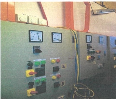
Figure 3.5: Air conditional panel
