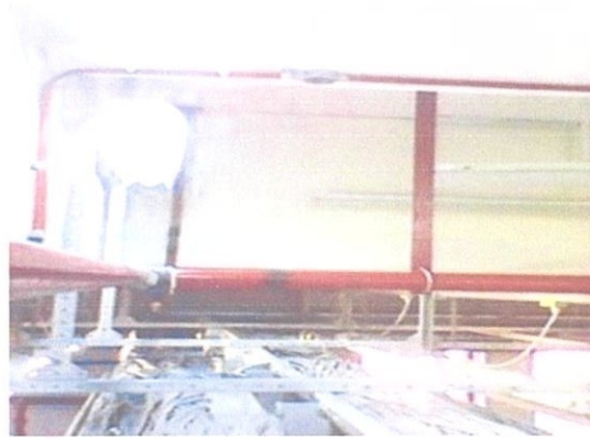
Figure 3.8: piping support with bracket
