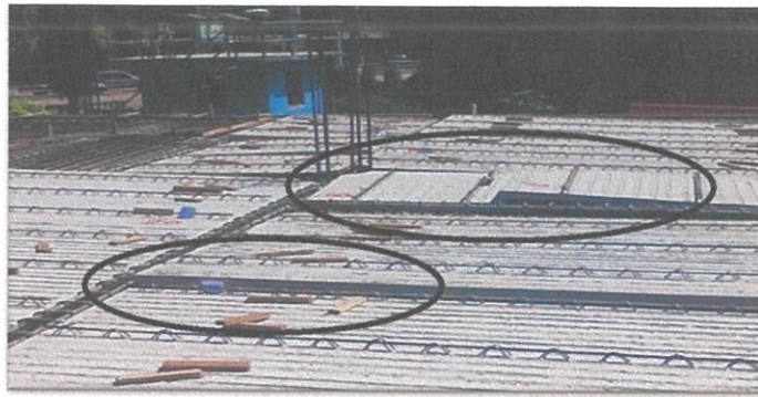
Photo 3.11 : The problem that found on the slab area
