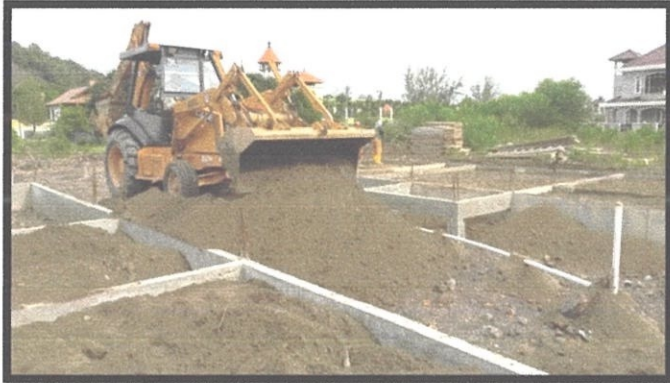
Photo 3.23 Cohesive soil were brought by bulldozer which be poured into floor slab
